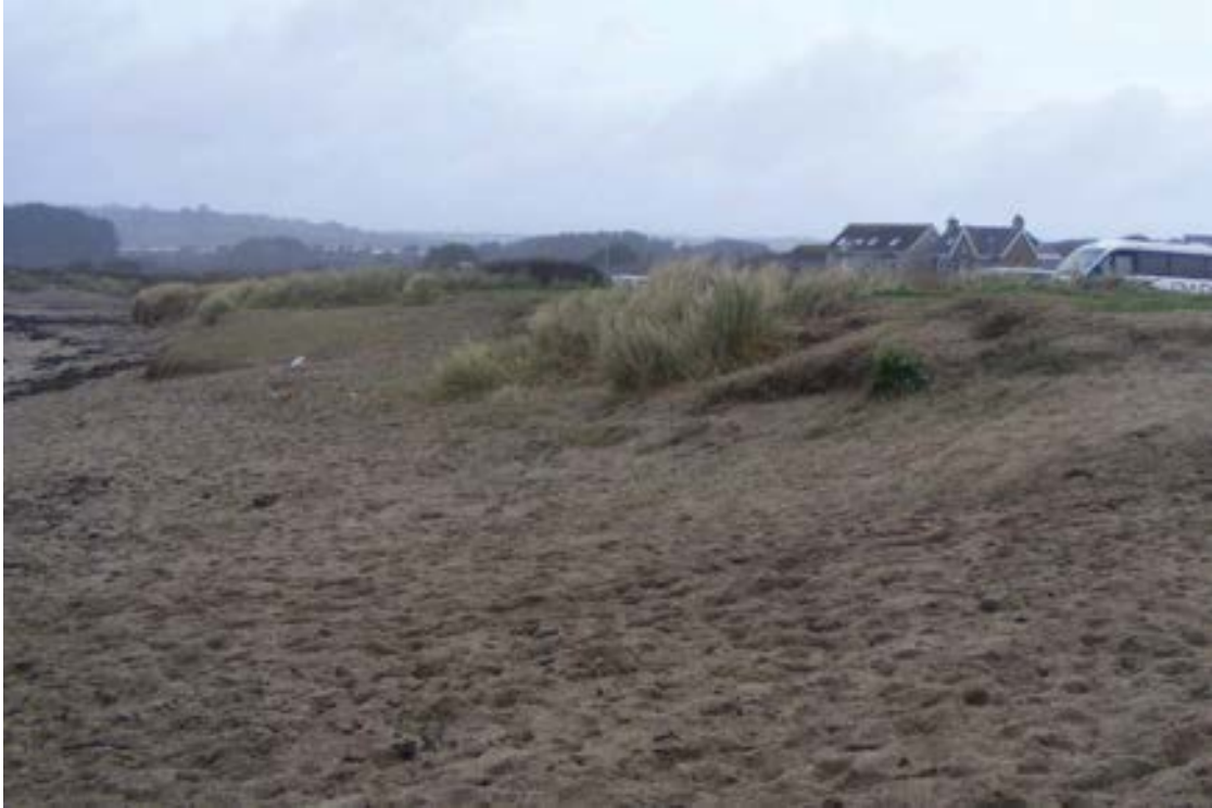
Figure A.11 Car park fronted by eroded dunes, with sandy beach (taken during site visit 1 st February, looking north west).
