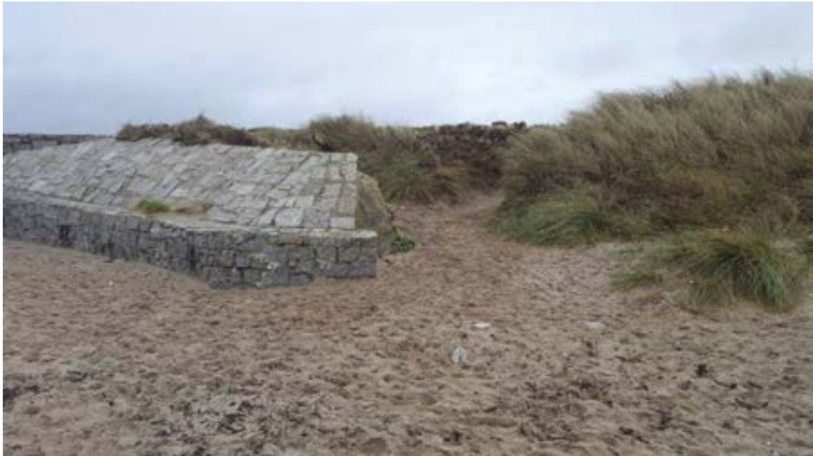
Figure A.3 Section to the west of Marazion where the seawall meets the dunes (taken during site visit 1st February, looking north- the Marazion Marsh is behind this defence). There are clear access issues here where members of the public use this section to walk from the road behind to the beach. This is potentially a weak point which could be vulnerable to breaching in the future.
