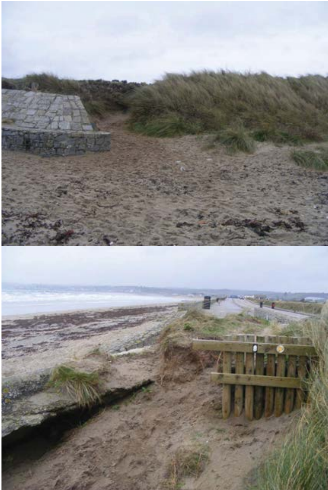
Figure 2.7 Western end of dunes where hard-defences start show clear signs of outflanking – an obvious weak point in the defence line.
