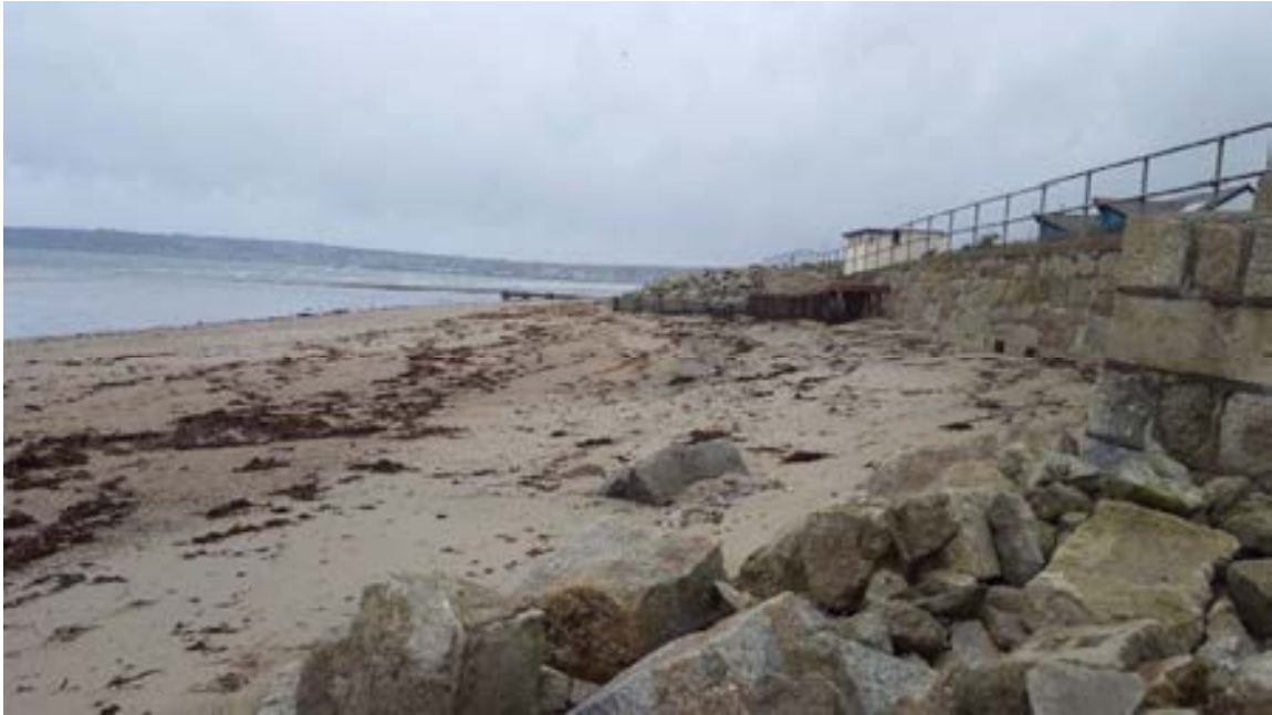
Figure A.1 Seawall and rock armour defences at Long Rock (taken during site visit 1st February, looking west towards Penzance). The outfall is visible in the background.
